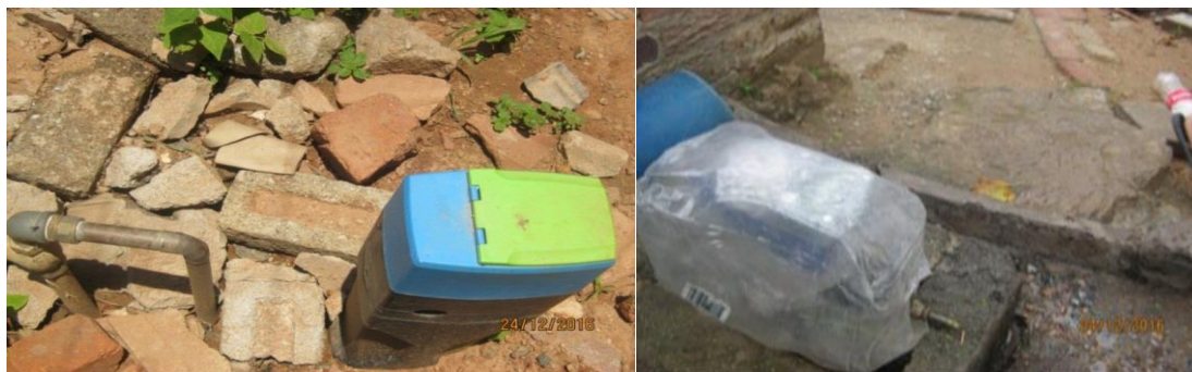
Figure 1: Prepaid water meters in Mabvuku, Harare
