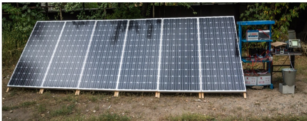
c) System for powering the ozonator with alternative energy through solar panels
